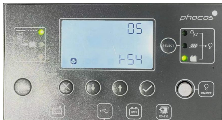
Figure 2.1.2.5 Phocos inverter battery type selection
