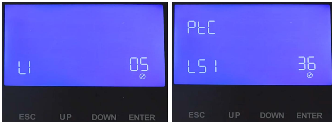
Figure 2.1.5.9 Growatt operation panel
